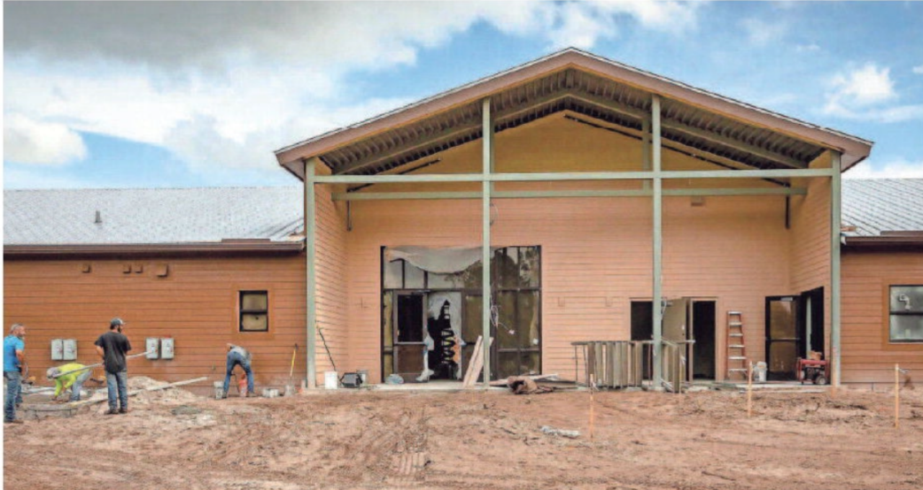
An east-facing view of the environmental education center as construction continues Thursday at the new Busch Wildlife Sanctuary in Palm Beach County. PHOTOS BY THOMAS CORDY/THE PALM BEACH POST
