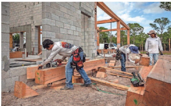
Beams are cut by a work crew at the education amphitheater during ongoing construction at the new Busch Wildlife Sanctuary.
